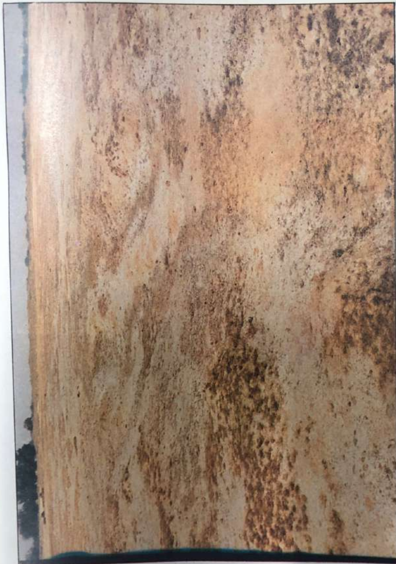
A view of salt affected area
